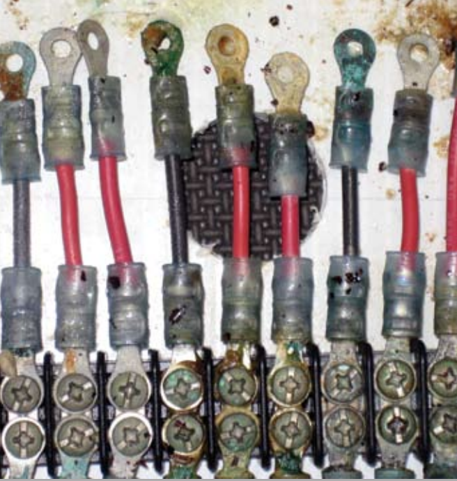
After six months, protection from the anti-corrosion sprays had worn off, but some greases still worked.
