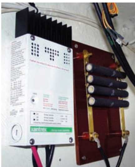
A Xantrex C40 charge controller regulated charging, and a diversion load from Hotwire Enterprises absorbed excess amps to prevent overcharging of the batteries.
