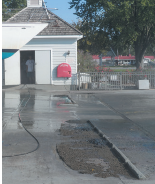
In order to meet local, state, and federal guidelines for runoff into adjacent waters, most boatyards are required to trap powerwash runoff to be sent out later for treatment.
