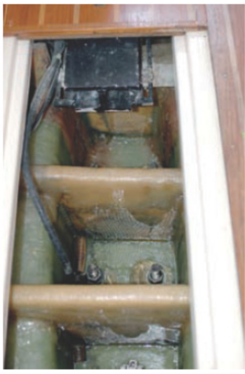
Fiberglass athwartship floor frames helped reinforce the keel stub and cope with the side force imposed by the lead ballast keel.
